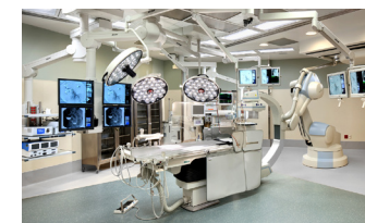
UK HealthCare Surgery Suite Lexington, Ky Full Architectural Services Collaborated with HGA
